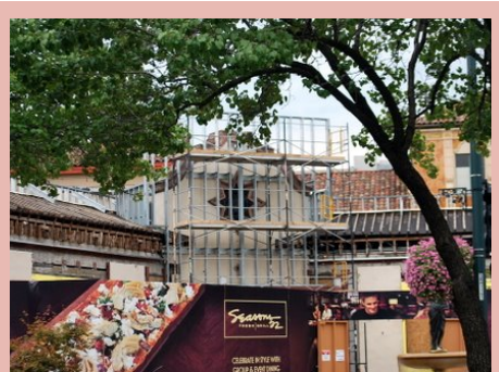
Retail space at Wornall and Ward Parkway under renovation with framing to cover the original architectural details. Seasons 52 has since decided to restore the facade, causing rejoice across the City. Photo by Mary Steeb.
